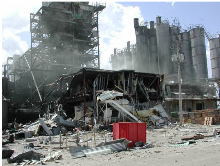
Figure 5. Damage to the Safety and Engineering offices
