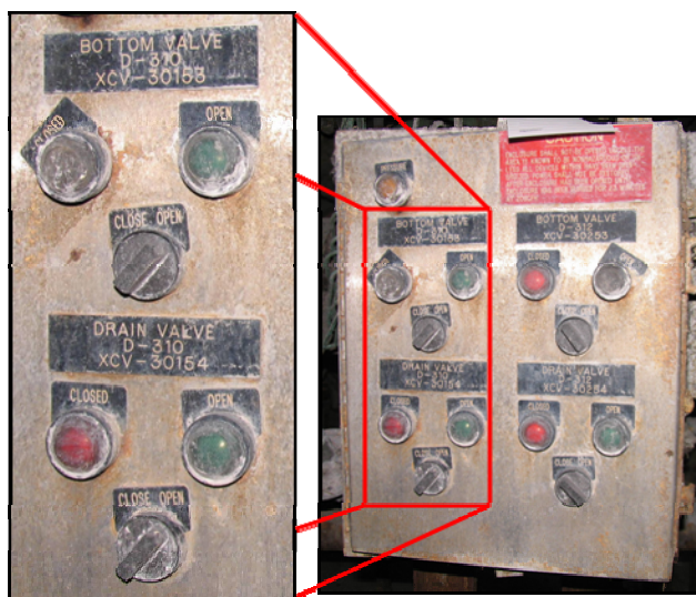
Figure 6. Reactor D310 bottom valve control panel as found after the explosion
